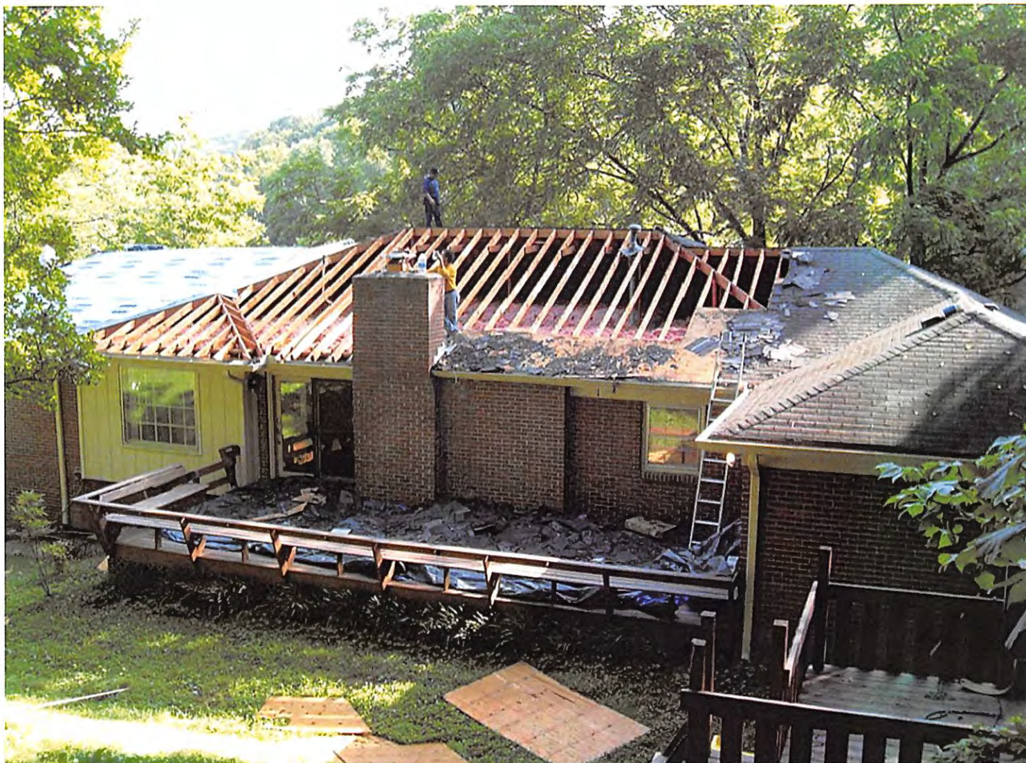
Right before the storm came through .... Two hard years of fighting, to get repaired and partially compensated.
